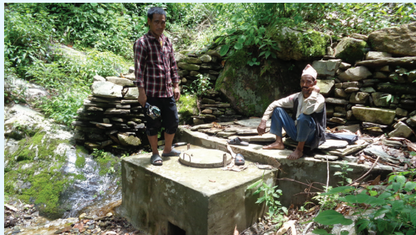
PHOTO 3: WATER INTAKE OF GHARIHOLA DRINKING WATER PROJECT
