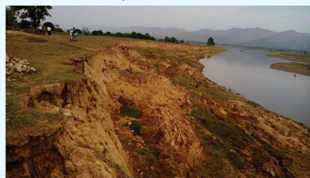
PHOTO 2: DAMAGED RIVER BANK PROTECTION WORK IN BELA VDC, DANG DISTRICT
