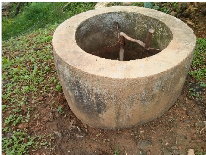
Fig. 5. Household level biogas plant. Source: Author.
